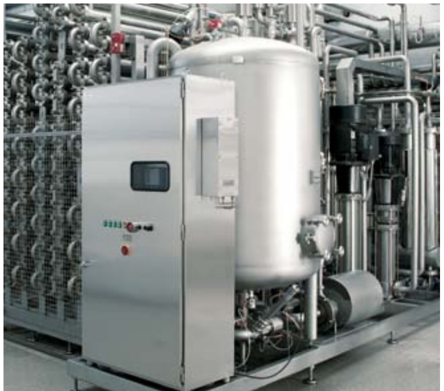
Indirect heating plant
