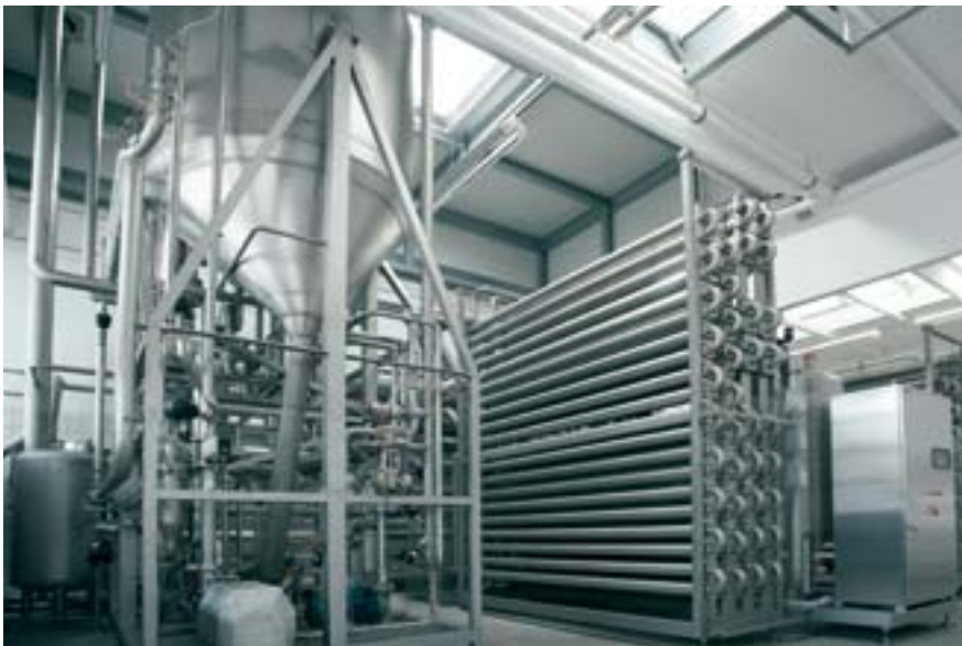
Direct heating plant. The photo shows tube modules and ash cooling unit.
