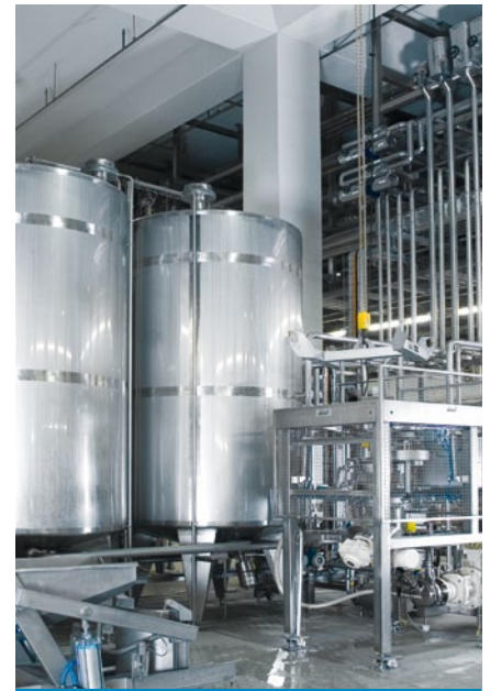
Powder mixing station
