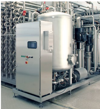
Indirect heating plant
