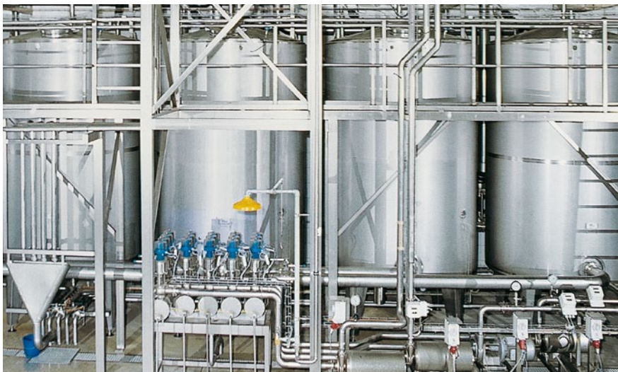
CIP batch cleaning assembly
