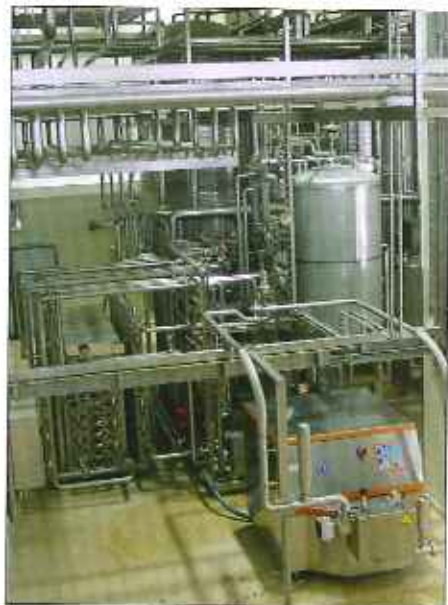
Each of the 4 pasteurisers has its own de-aerator and homogeniser
